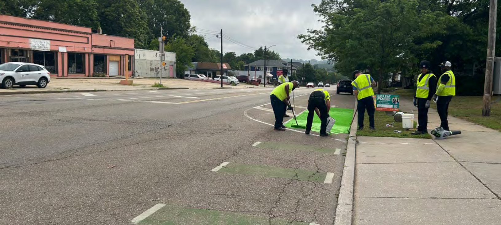
City workers apply new paint to the project. Source: City of Akron.
